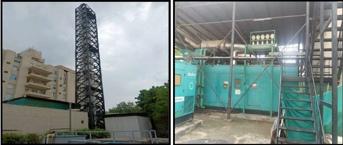
Photograph:- D.G Set with Acoustic enclosure and Adequate Stack Height
