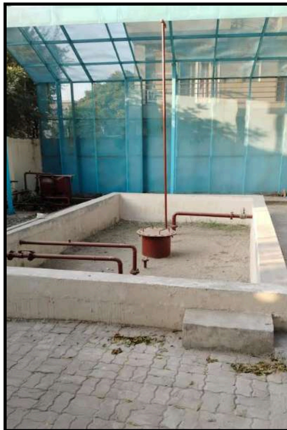
Photograph :- Fuel storage area
